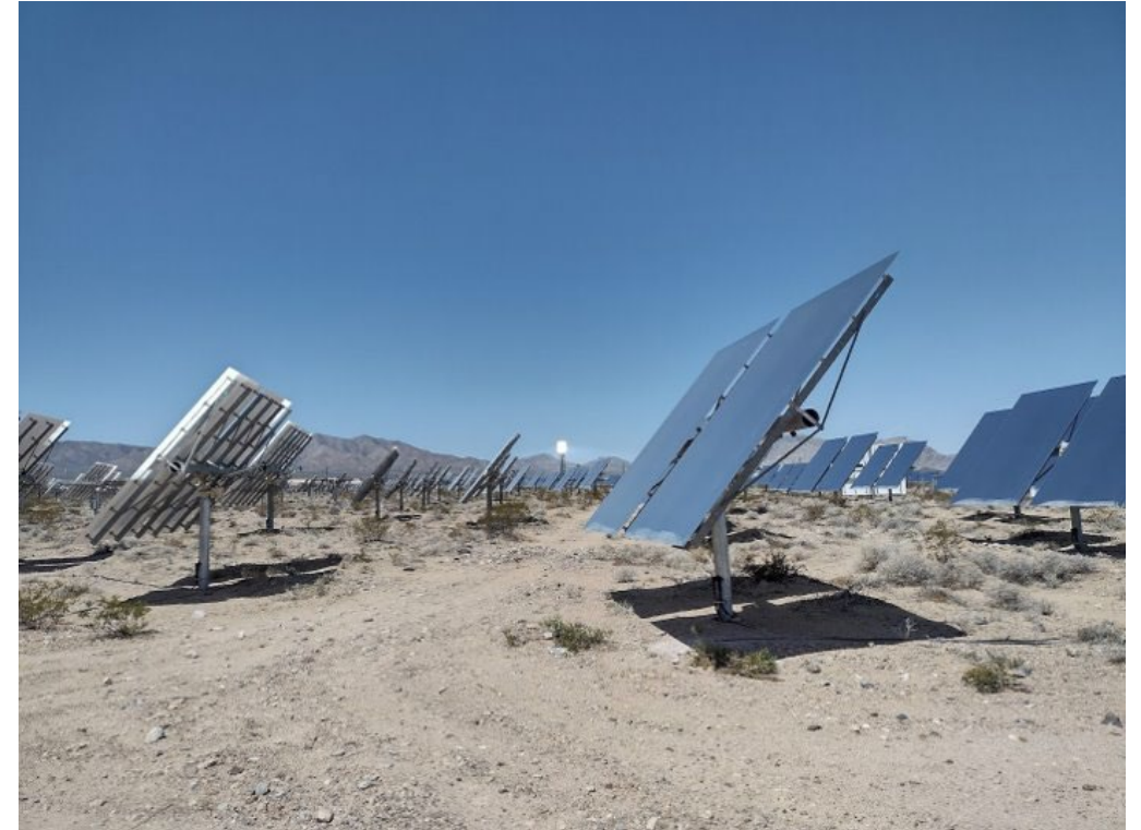
Heliostats in Solar Field 1 of Ivanpah Solar Generating Facility
