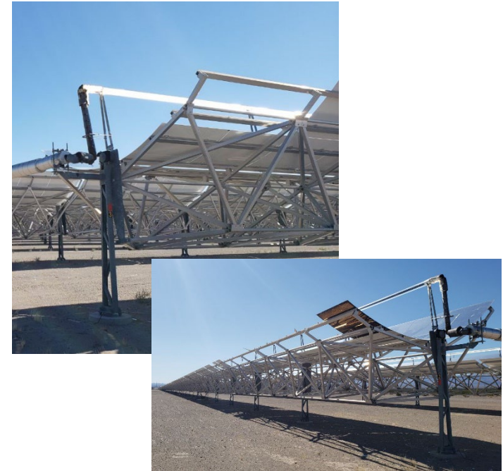
Parabolic trough rows at the Nevada Solar One (NSO) solar power plant with damaged mirrors on the outer edge of the field. Photos by Ulrike Egerer, NREL
