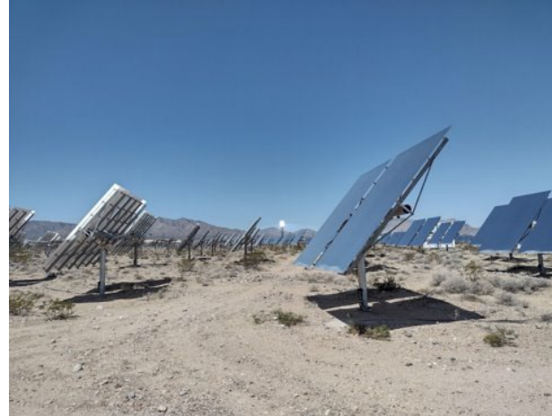
Heliostats in Ivanpah Solar Field, Unit 1
