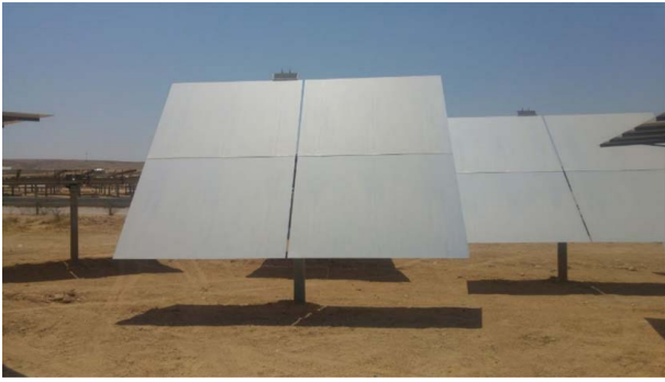
Fig. 7 Wireless BrightSource heliostat at Ashlim with top-mounted PV panel. A small heliostat is estimated to consume less than 1 kWh per day [69]. Heliostat-attached PV panels can therefore provide feedback data and eliminate power cabling. Adapted from Ref. [51].
