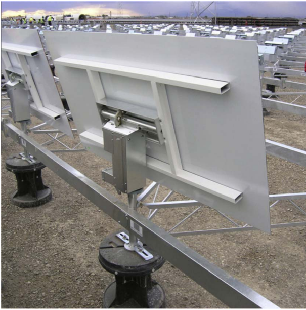
Fig. 4 eSolar trussed and ballasted heliostat 24,000 mirror modules mounted on shared trusses are used at the SunDrop facility. The diminutive heliostat represents a design approach that focuses on minimizing cost of installation at the site; according to eSolar, installation used local unskilled labor, with only one size of wrench needed for complete assembly. Adapted from Ref. [3].
