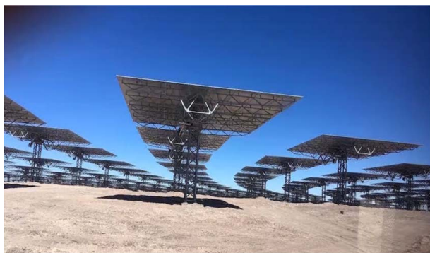
Fig. 3 Abengoa trussed heliostat at Atacama I. This design eliminates torque tubes entirely. This can lower the structure's cost in two ways. First, less material (by mass) is used. Second, there is no need to separately procure and process a small quantity of one specific tube/pipe size for the torque tube. Adapted from Ref. [37].
