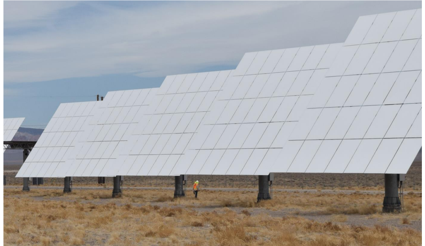
Crescent Dunes Heliostats
