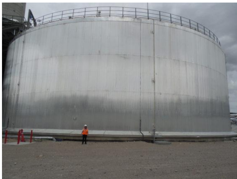
Figure 9: A molten salt tank for thermal energy storage [d]
