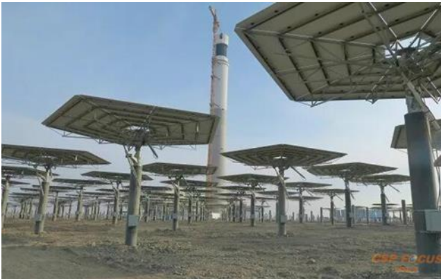
Figure 15: Pentagonal Heliostat Supports, Hami [h]
