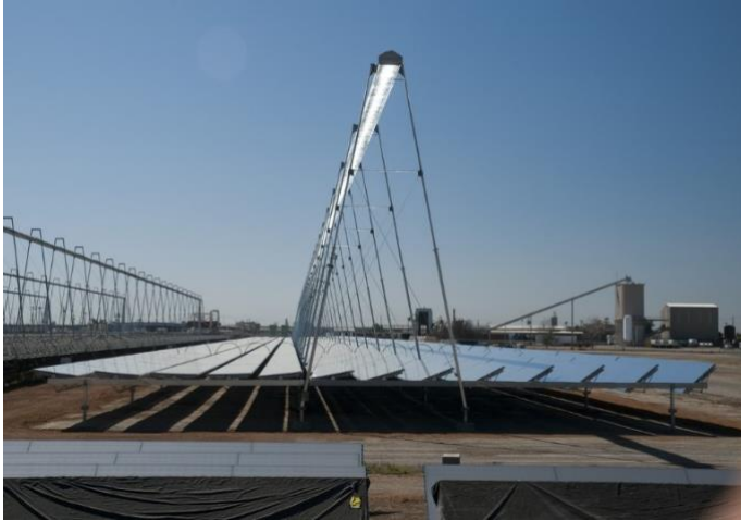
Figure 3: Linear Fresnel collectors at Kimberlina Solar Thermal Power Plant
