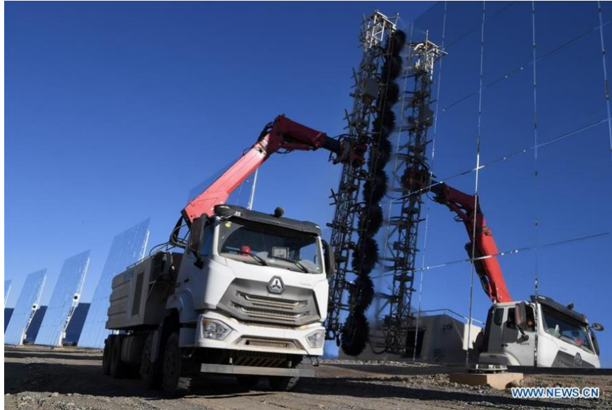
Figure 27: Semi-automatic heliostat cleaning [s]
